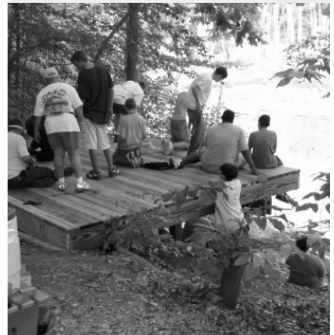
Boy Scout Troop 870 constructs the Beaver Pond observation platform for Steve Medina's Eagle Scout project.
